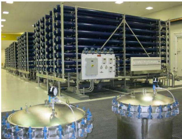
North RO Plant Production Trains
